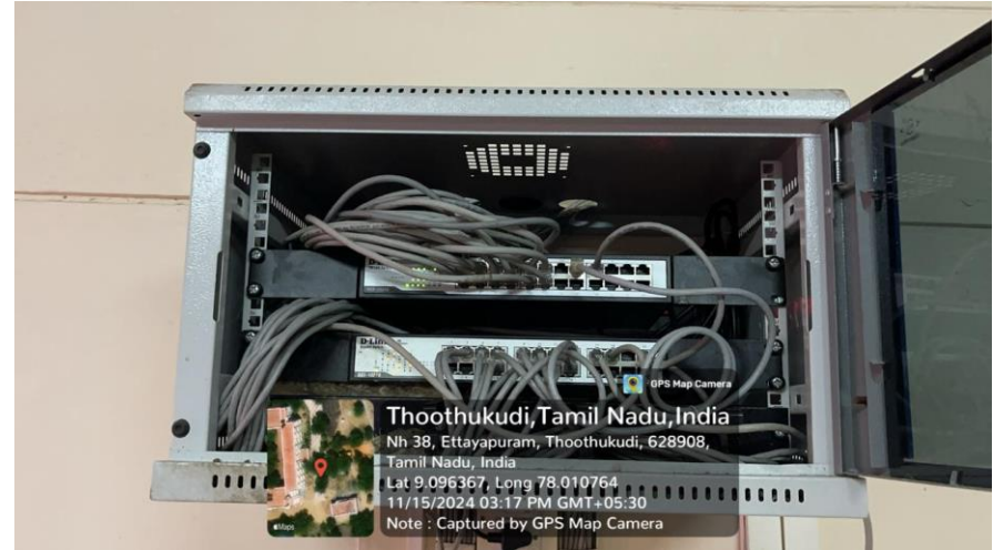
Computer lab 2 Network Switch2
